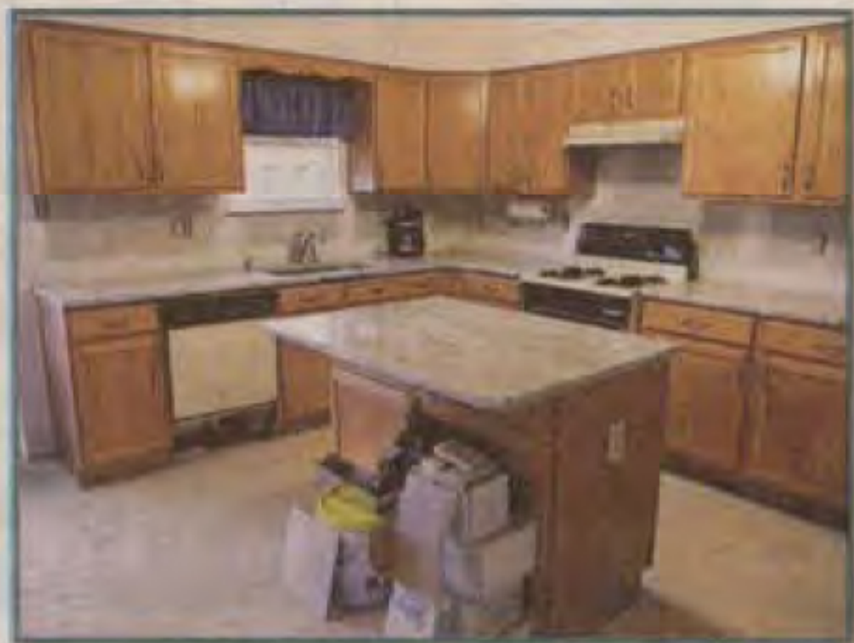
The Berlin Borough kitchen of Kristin Braidwood and Len DiGiacomo is a work in progress. Renovation includes floor, backsplash and countertops.
